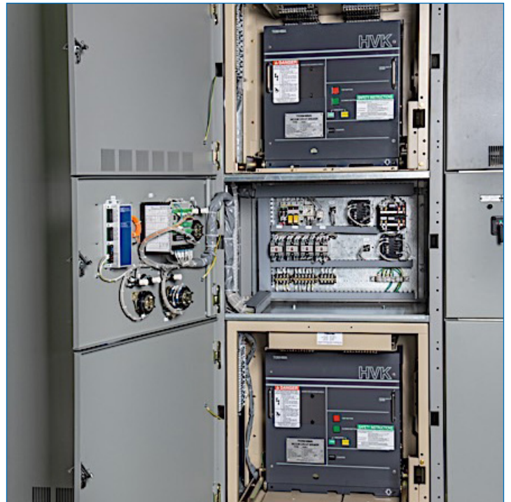
Two OEM Cells Installed in a 95 in. High Metalclad Switchgear (5 kV/15 kV Rated)
