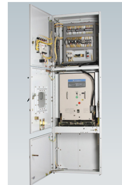
Figure 4-1 Front compartments of MS-E (switchgear)
