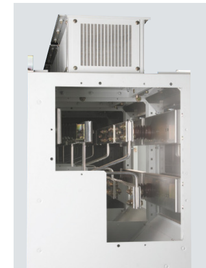
Figure 4-2 Main busbars (air-insulated) with tin plating
