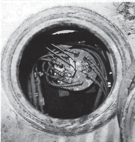
Manhole, drop thru access, remote mechanical switching with VACop IV operator. Mechanical operator (top photo) with drop through access into vault (bottom photo).
