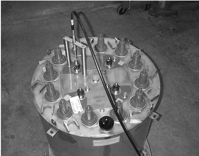
Figure 14. VACop IV operator attached to VACpac switchgear.
