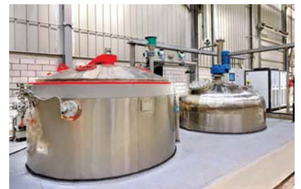
Vacuum pressure impregnation plant
