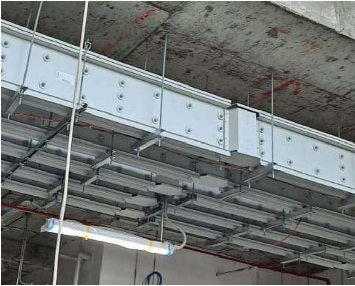
Example of Bahra busbar system
